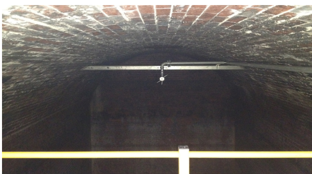
Storm Blaster installed in a covered tank
